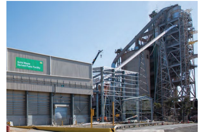
Alternative fuels facility at Berrima, NSW
